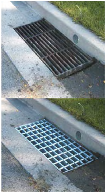
Figure 10 - Above, poor drainage grate choice; Below, bicycle-friendly grate (photos courtesy of Syrcast)
