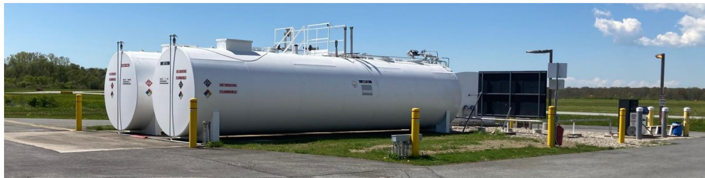
Figure 1-6: GFL Fuel Tanks
