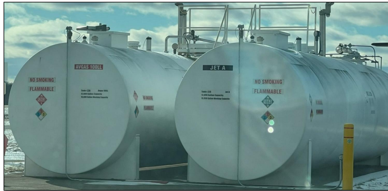
Figure 2-2: GFL Fuel Tanks
